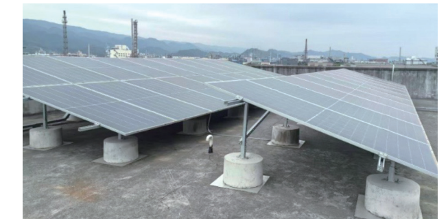
Solar power generation that started in November 2025 at the Chongqing site
