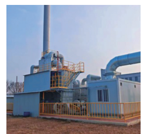
VOC treatment equipment at the Tianjin site
