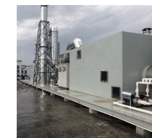
VOC treatment equipment at the Zhongshan site
